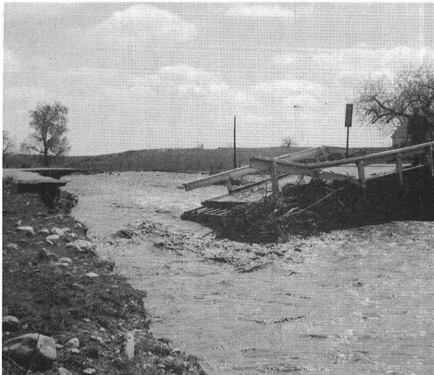
County Bridge at Dillon Road, washed out.
