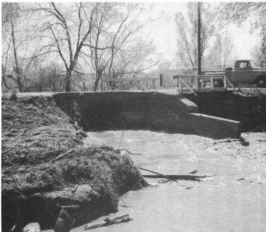
Bridge approach in town of Superior, damaged.
